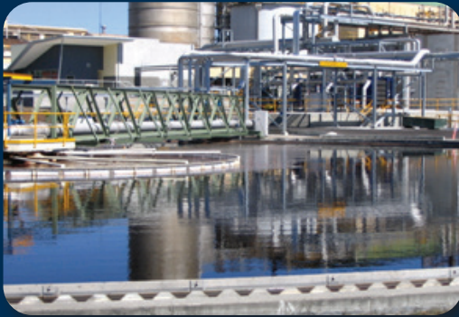
Clarifier — Pulp and Paper Tasmania
