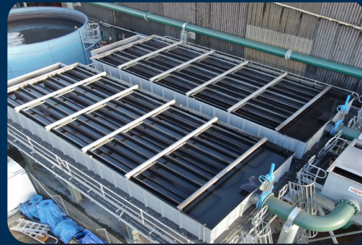
Lamella Clarifier — Steel Manufacturing New Zealand
