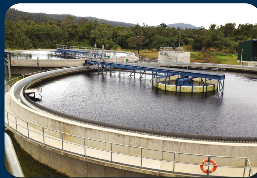
Clarifier — Municipal STP Queensland
