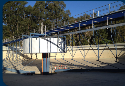
Clarifier — Municipal WWT New South Wales
